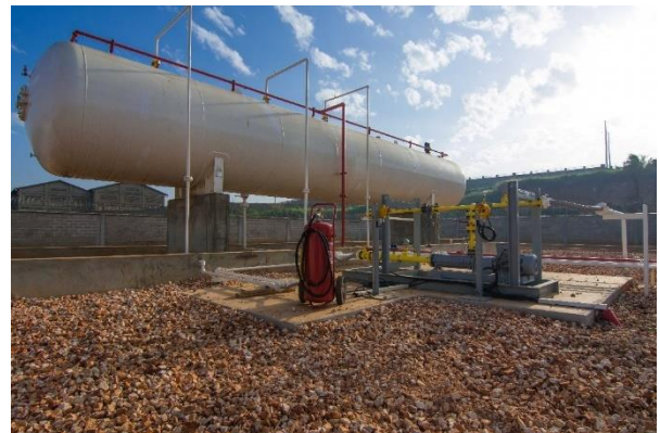
LPG bulk storage facility
