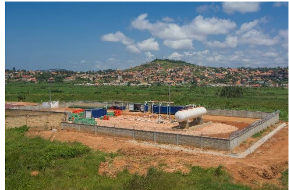
Overview of a containerised filling facility
