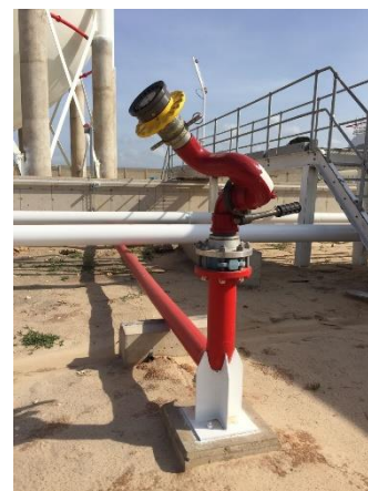
Fire water nozzle
