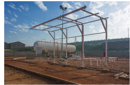
Road tanker unloading bay with fire water system
