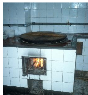
Figure 1.3a - Wood fired stove in commercial kitchen
