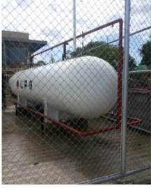
Figure 1.3f - Small above ground bulk tank
